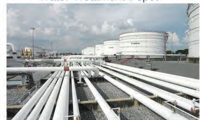
Jet Fuel Pipeline
