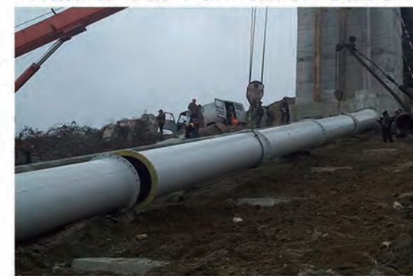
Slurry Conveyance Pipeline
