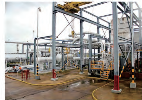
Natural Gas Purification Station
