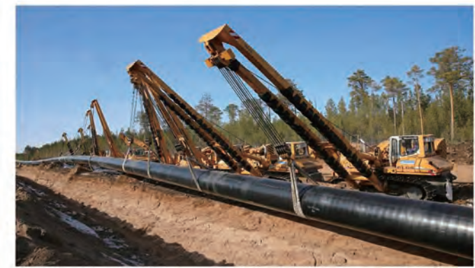
Crude Oil Pipeline
