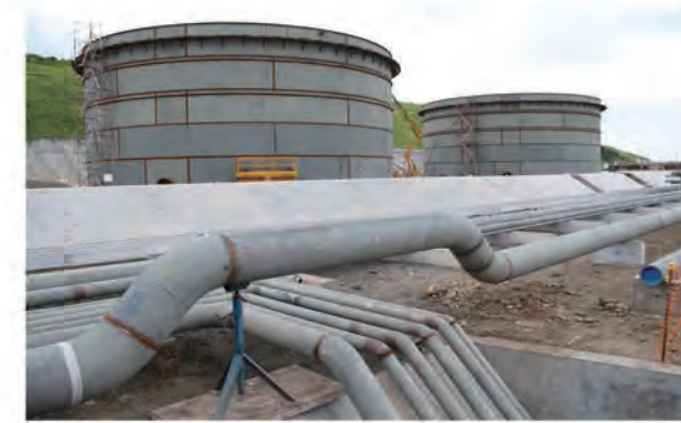
Oil Storage Terminal
